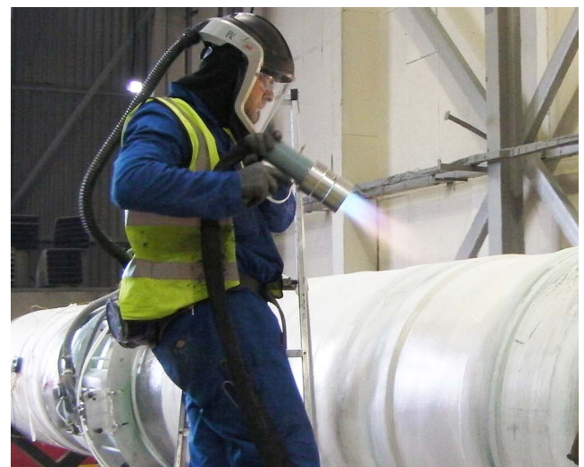
The above field joint is being flame spray coated with Plascoat® PP10.
